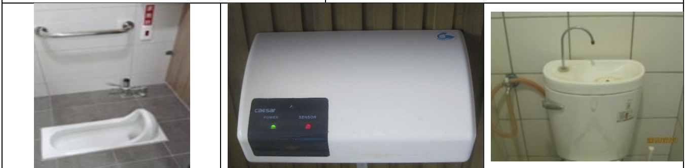
Induction faucet and installation of water-saving device
