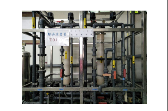
Recycled Water Filtration Equipment
